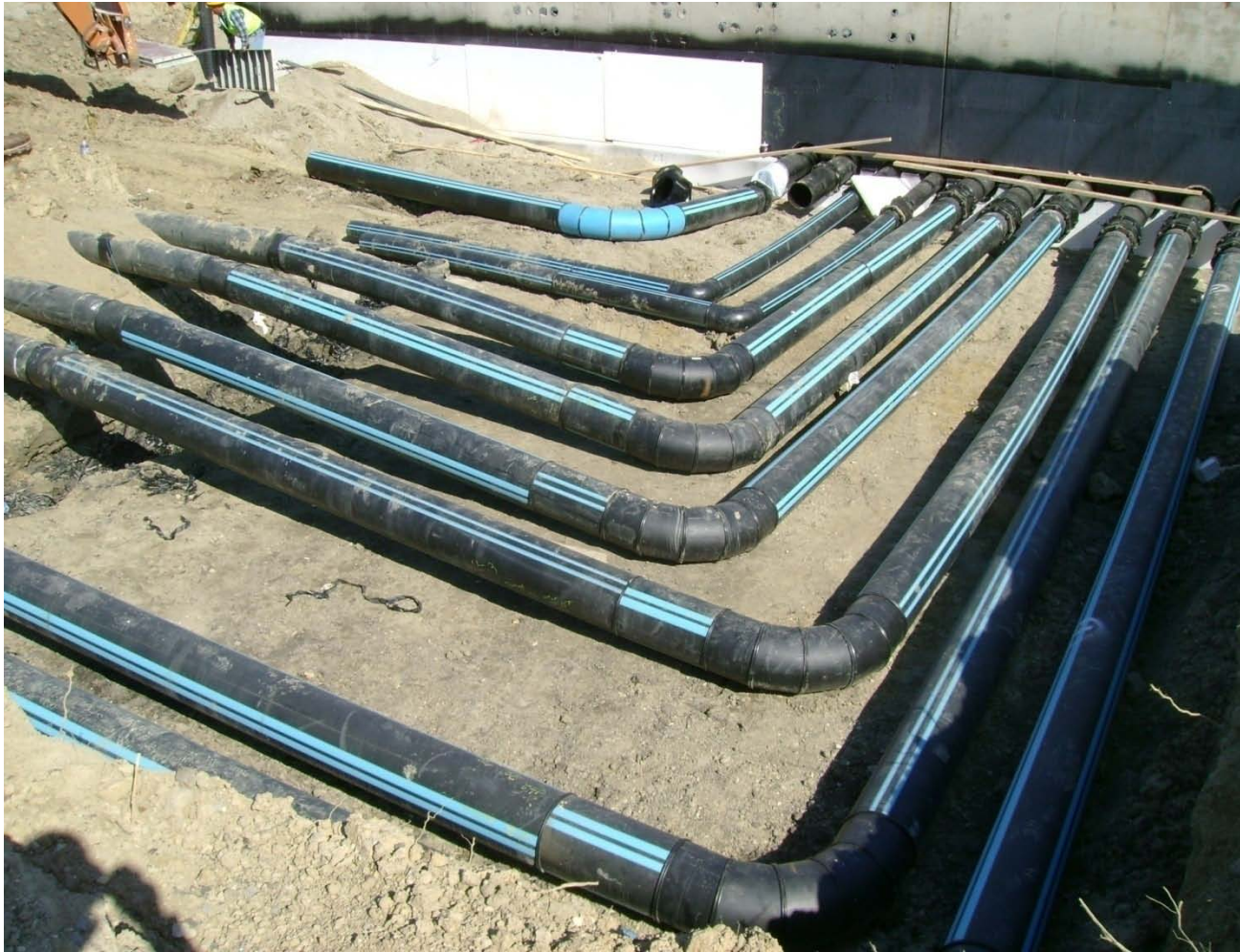
Loop Field Headers 16,000 to 20,000 GPM
