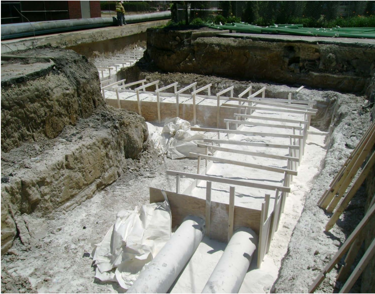
10 miles of hot water supply and return pipe
